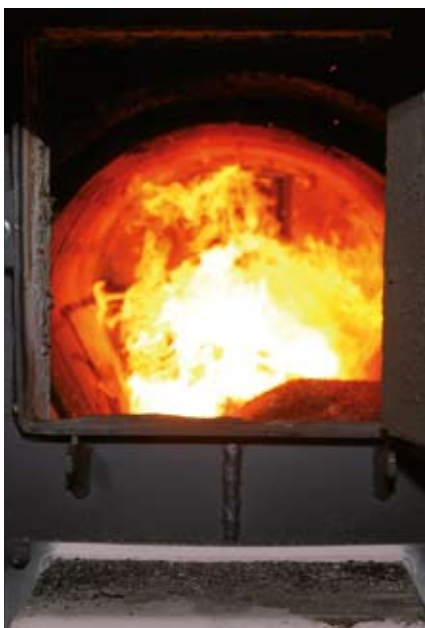
Burning wood chips - A view into the boiler
