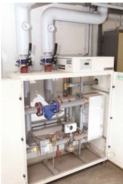
A district heating substation in the Wiesmath community
