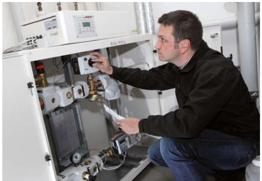
The responsible sales engineer from Danfoss – Martin Stocker – looking at a heating system installed in a nearby school
